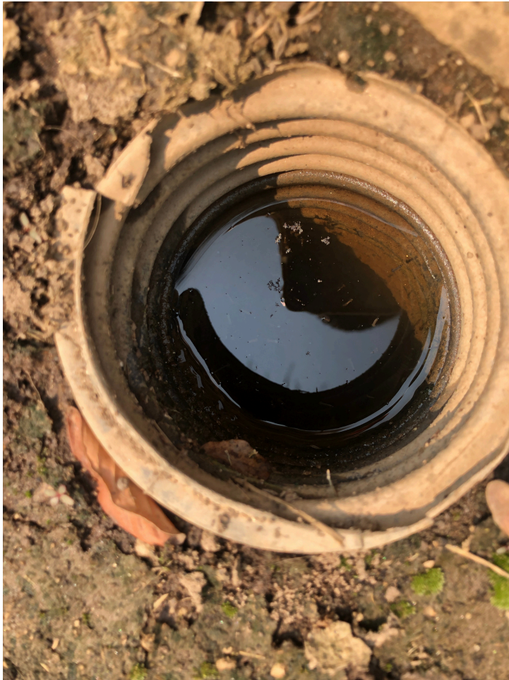
Yard drains that are not properly screened and capped are among the most frequently identified sources during service requests.
